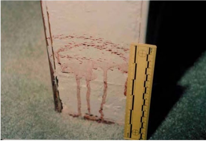
Figure 8.16 Base of doorjamb with laterally oriented projected stains; note downward flow patterns. (Courtesy of Rex Sparks, Des Moines, Iowa Police Department.)
