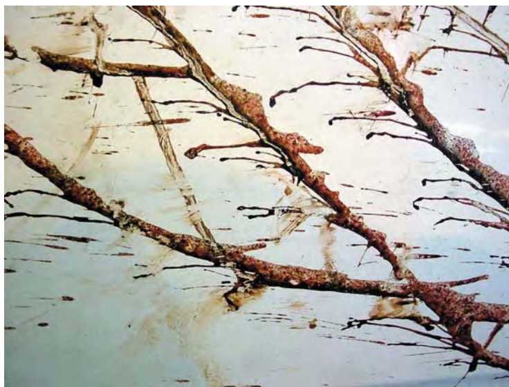
Figure 13.44 Closeup view of the stains described in Figure 13.43.
