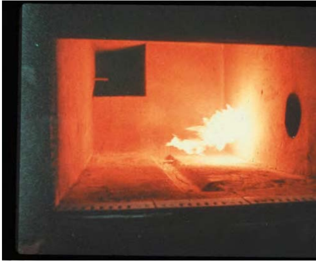
Figure 9.34 View of improperly working flame port in Furnas.
