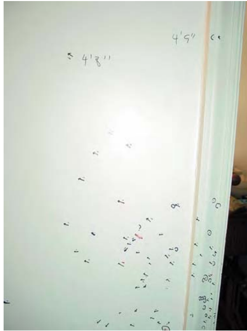
Figure 10.22 Void to left of door facing.
